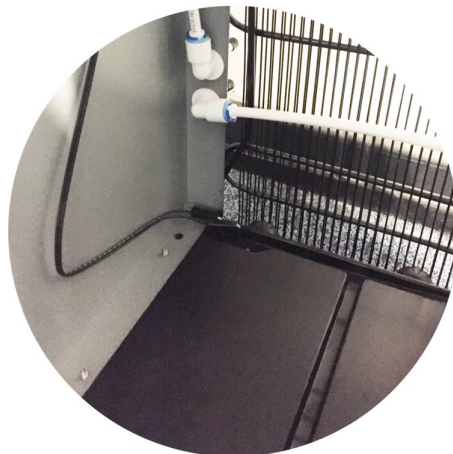
Photo Flood probe located on the base floor of the technical compartment
